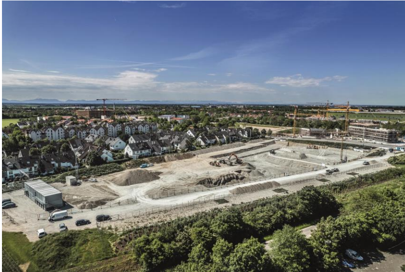
(1) Construction of an excavation pit in the town hall district of Kirchheim near Munich
