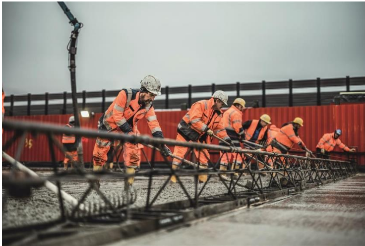
(2) Placing of concrete in front of the vibrating beam for construction of the concrete surface.
