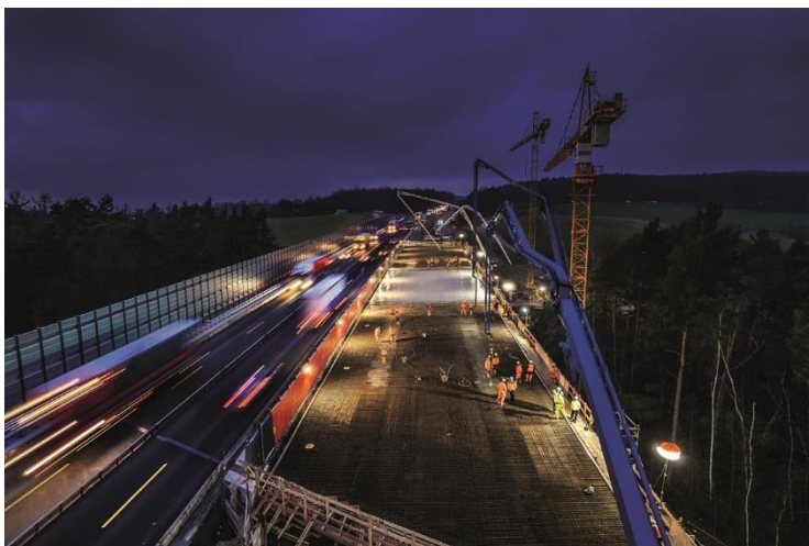
(1) A feat of strength: Concreting work for the superstructures of the second construction section of the Innerstetal bridge was carried out in just one day.
