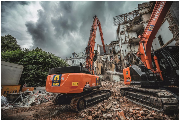
(1) The environmental division of BAUER Resources GmbH was tasked with the demolition of a 1950s residential building in the Lehel district of Munich.
