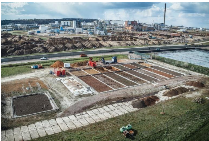
(1) In 18 successive filter basins, the Bauer Umwelt groundwater treatment plant in Leuna cleans contaminated water with the help of microorganisms using a purely biological method.
